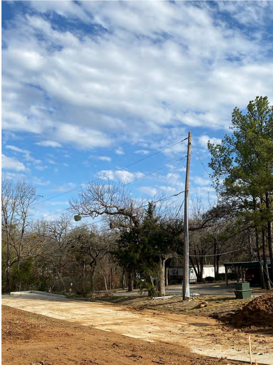
Westernmost Pole on Adjacent Property – Pole Transformer and cable lines exclusively serve adjacent property.
