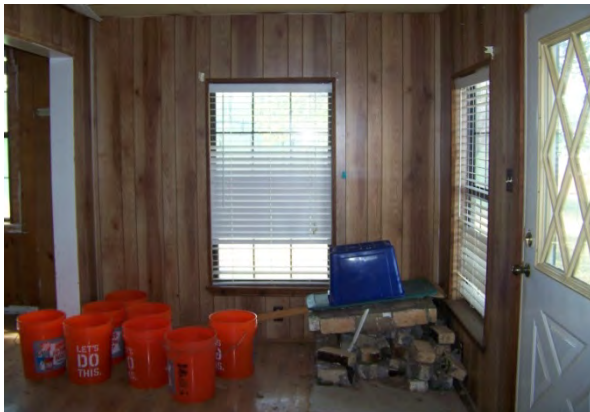
Interior view of the Utility room looking south
