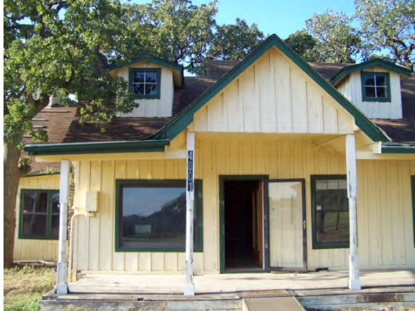
East portion of front porch leaning, column and floor damage
