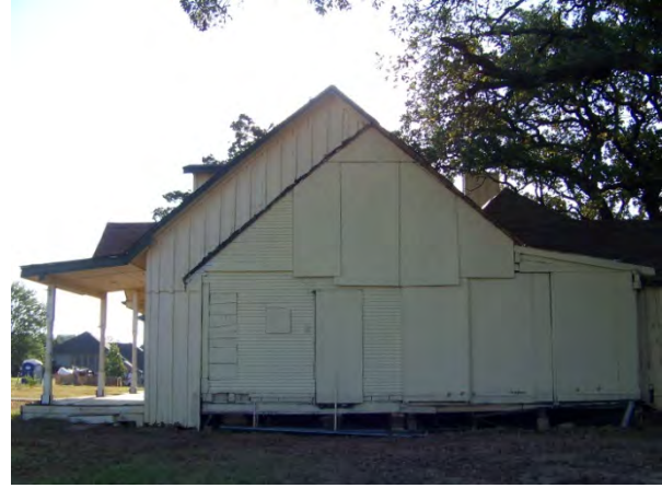
West elevation showing various layers of siding
