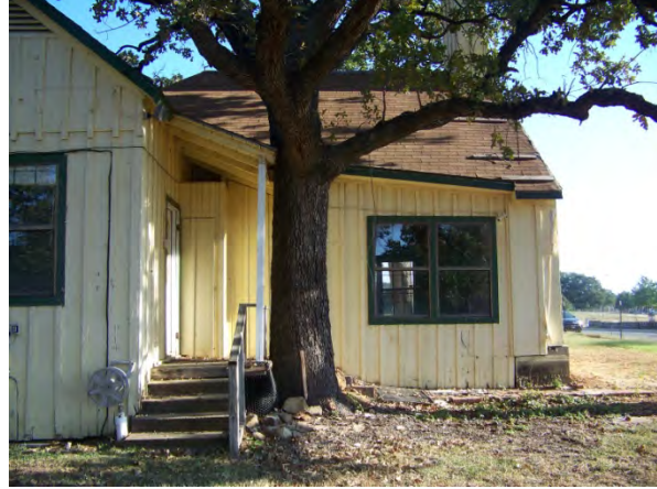
Existing roofing held down by wood and other materials.
