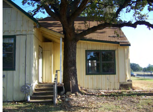
Rear porch leaning toward the house and tree encroaching
