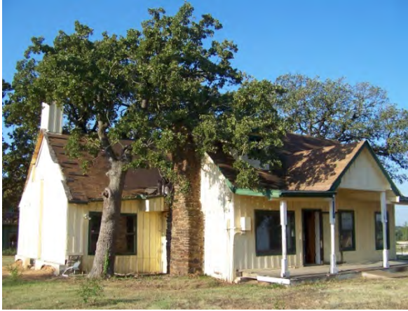
Existing roofing held down by wood and other materials.
