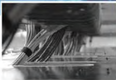
STRUCTURED CABLING | INFRASTRUCTURE MAINTENANCE
