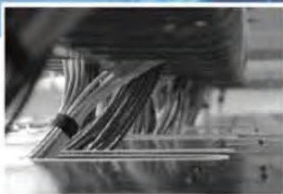
STRUCTURED CABLING | INFRASTRUCTURE MAINTENANCE
