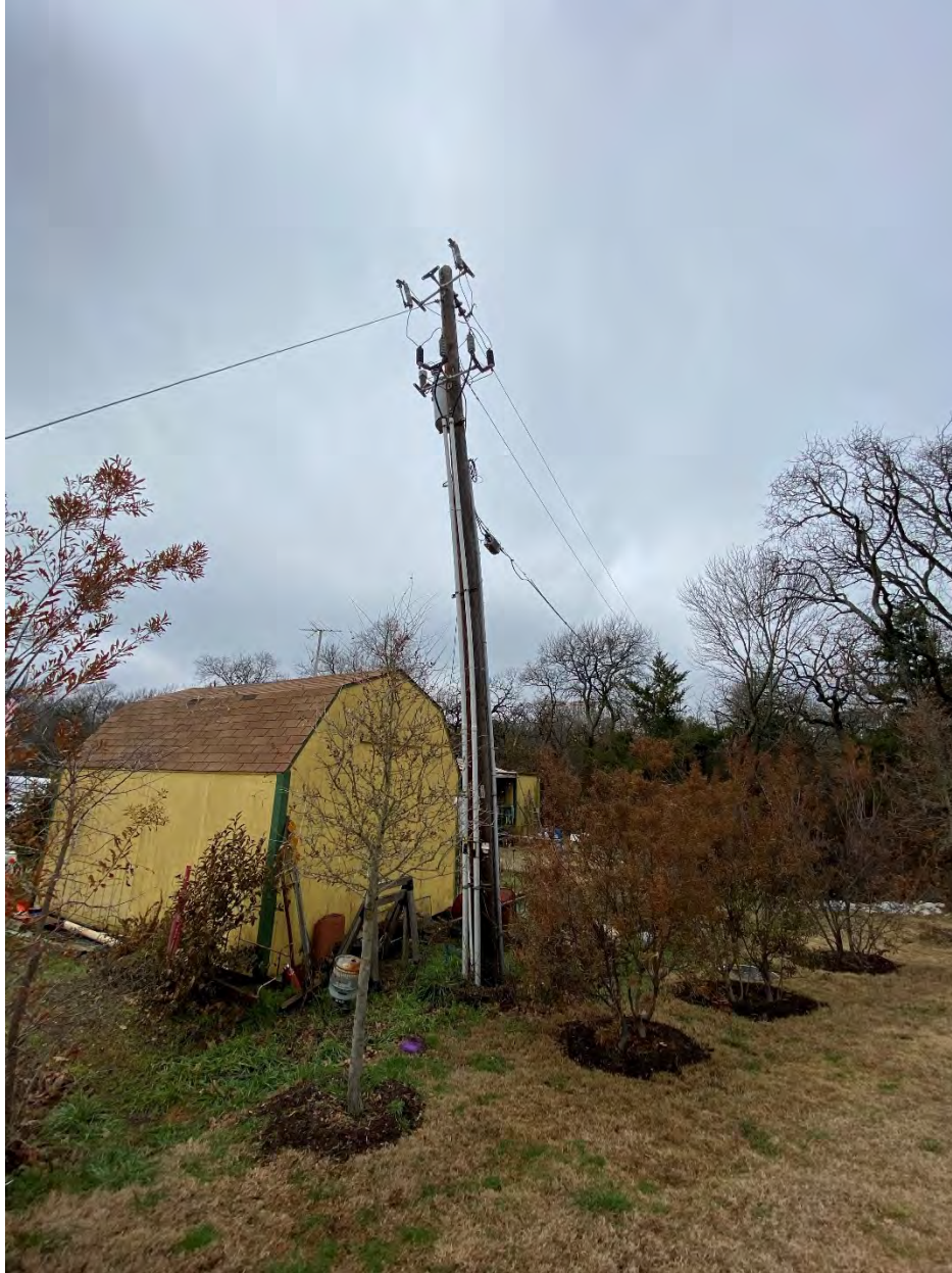
Easternmost Pole on Adjacent Property. Pole Transformer exclusively serves adjacent property.
