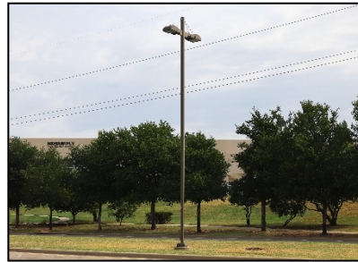
Example of existing light fixture
