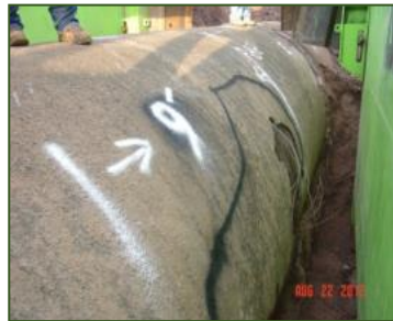
Damage concentrated in 9' section
